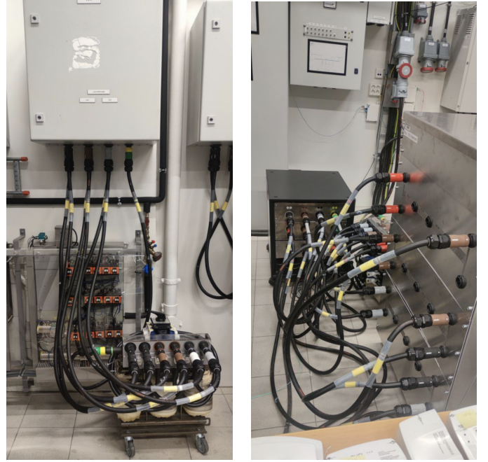
Fig. 3: Laboratory implementation of series and parallel RL circuits at SINTEF facilities.
